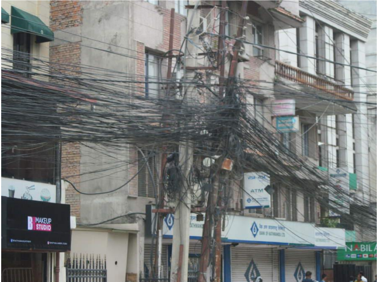
Jumble of wires on Kathmandu telephone pole
